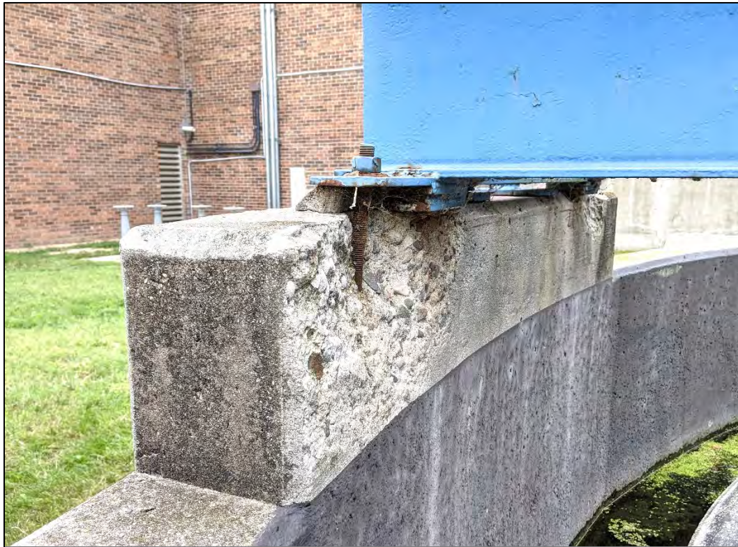
Figure 4 – Deteriorated Bridge Beam Support (with exposed anchor bolt)
