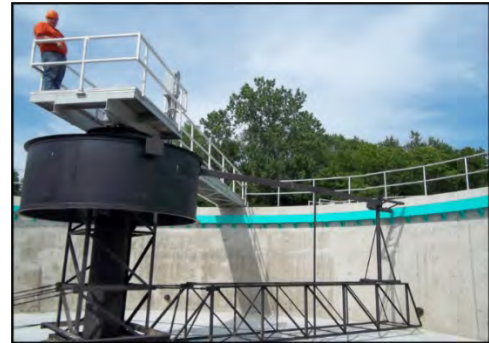
One of Several New Final Clarifiers & Mechanism
