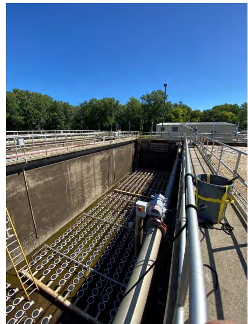
Aeration Tank “Flex Zones” with Large Bubble Nozzles and Existing Diffusers
