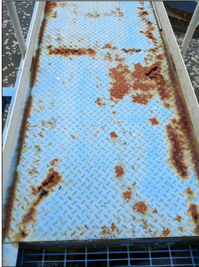
Figure 3 – Deteriorated Bridge Decking
