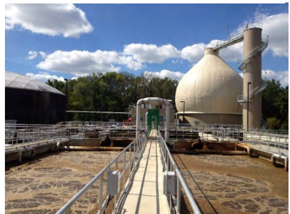
Egg-Shaped Anaerobic Digester and New Aeration System
