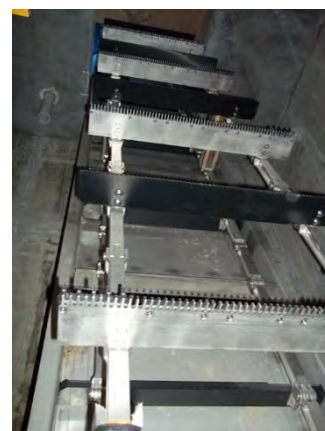
New Fine Screen Rakes Screenings to Surface Level Washer/Compactor
