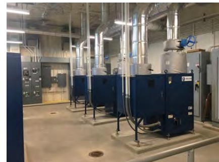
Blower Room with Control Panels
